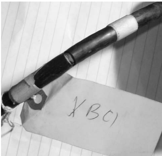
Fig. 6. XLPE 2-wire insulation cut. (wide cut to outer jacket with cut to conductor of each individual).
