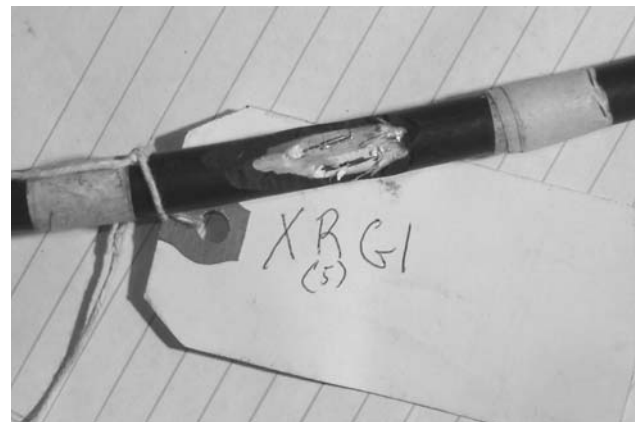
Fig. 8. Gouge through the outer jacket and through the XLPE insulation of two conductors.
